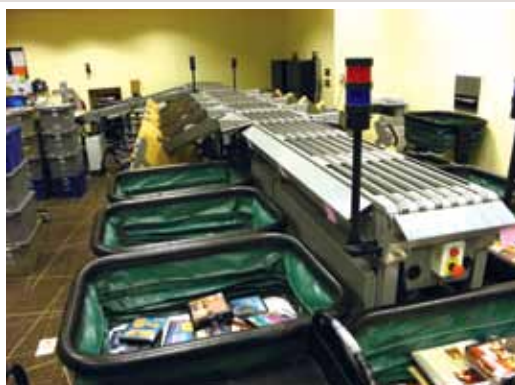
Automated Materials Handling System
